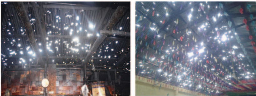
Fig. 1 Hail damaged galvanised iron sheet roofings
