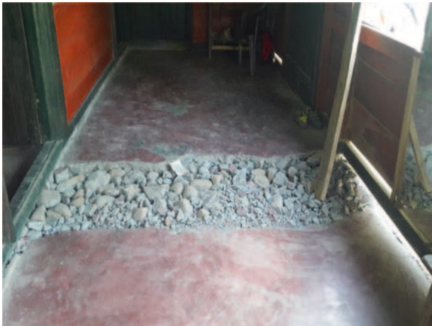
Fig. 6 An earthquake affected house in Noney
