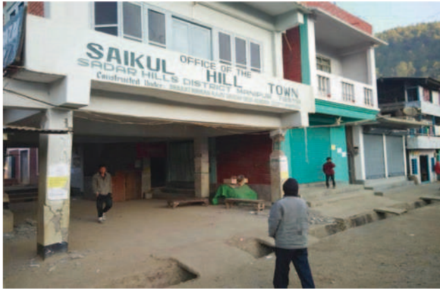
Fig. 5 Pillars of the office of the Saikul Hill Town developing cracks after 4th January Manipur earthquake
